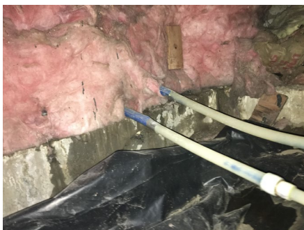
Water entry through cold joint
