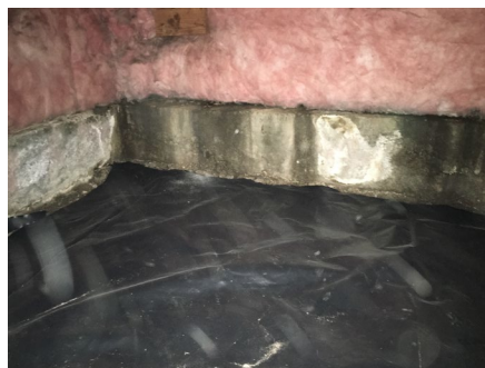
Water entry through cold joint
