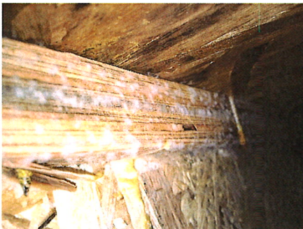
Mold on floor joist
