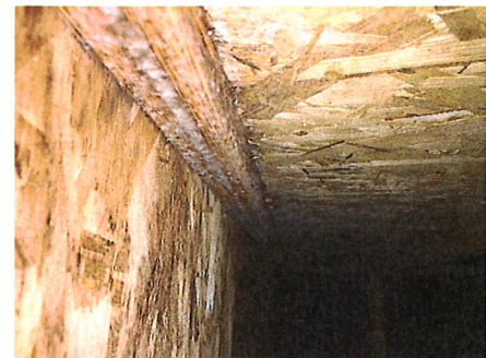
Mold on floor joist
