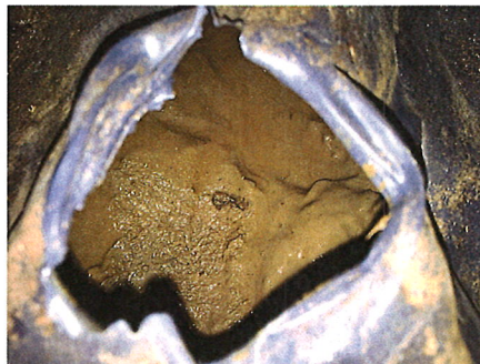
Wet/standing water under vapor barrier
