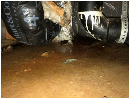
water in crawl under furnace
