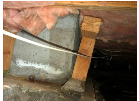
water damaged pony wall- side view- tilted
