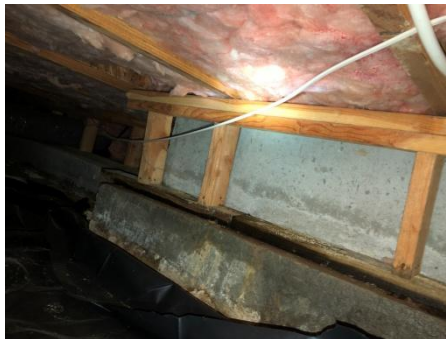
water damaged pony wall-front view
