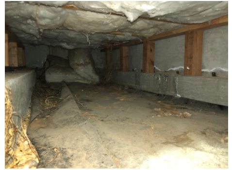
debris in crawl and hanging insulation
