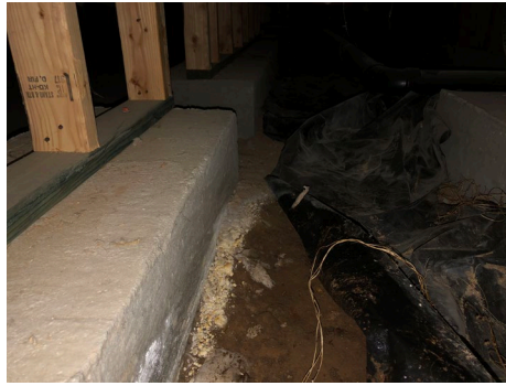
damaged plastic-not pulled up on footing
