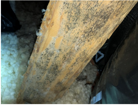
visible mold in attic
