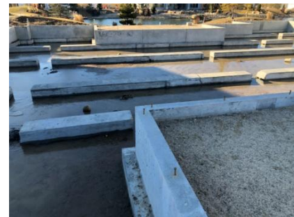
Adjacent property showing standing water
