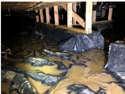
Standing water in the crawlspace
