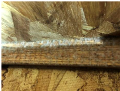
Microbial growth on top cord of floor joist
