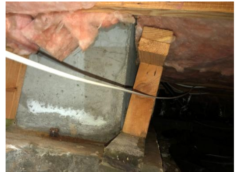
water damaged pony wall- side view- tilted
