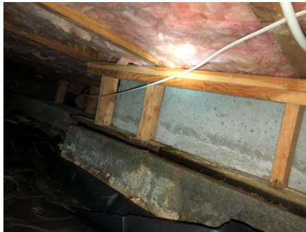
water damaged pony wall-front view
