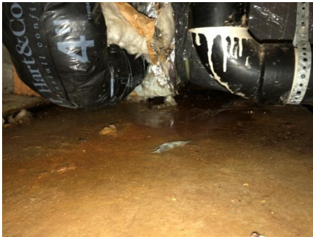
water in crawl under furnace
