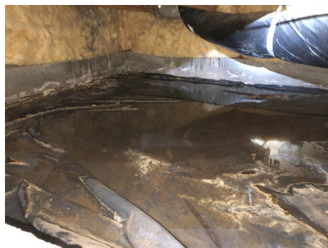
Standing water/Poor vapor barrier
