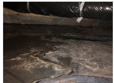
Standing water/Poor vapor barrier
