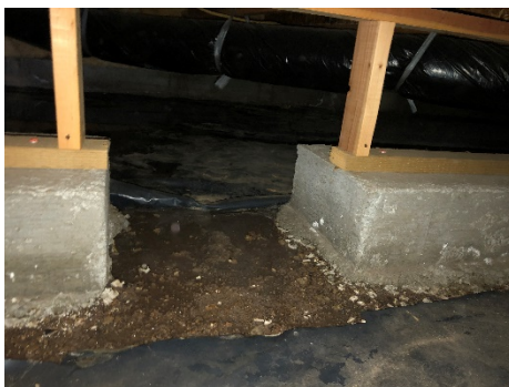
Water intrusion/Poor vapor barrier
