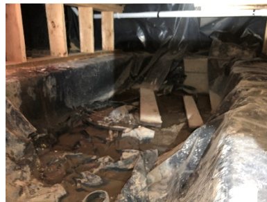
Standing Water/Poor Vapor Barrier
