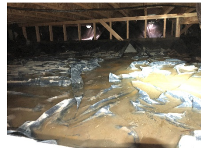
Standing Water/Poor Vapor Barrier
