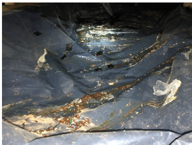
Standing Water on top of plastic
