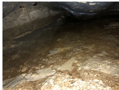
Standing water under the plastic
