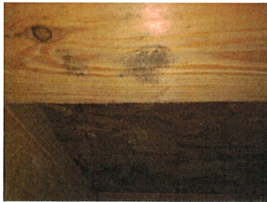
Mold growth on joist
