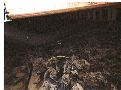
Vapor barrier in poor condition
