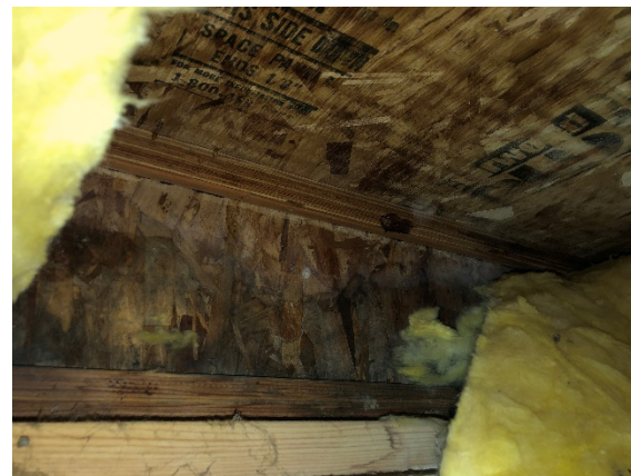
mold on the rim joist
