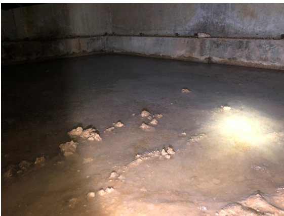
1.5 ft standing water in the crawlspace
